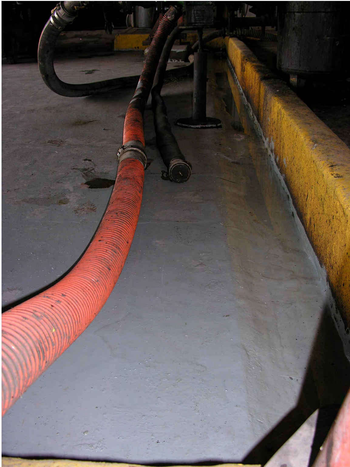
Unloading Area #1 Sump Trench at East End Showing Maintenance Recoat
