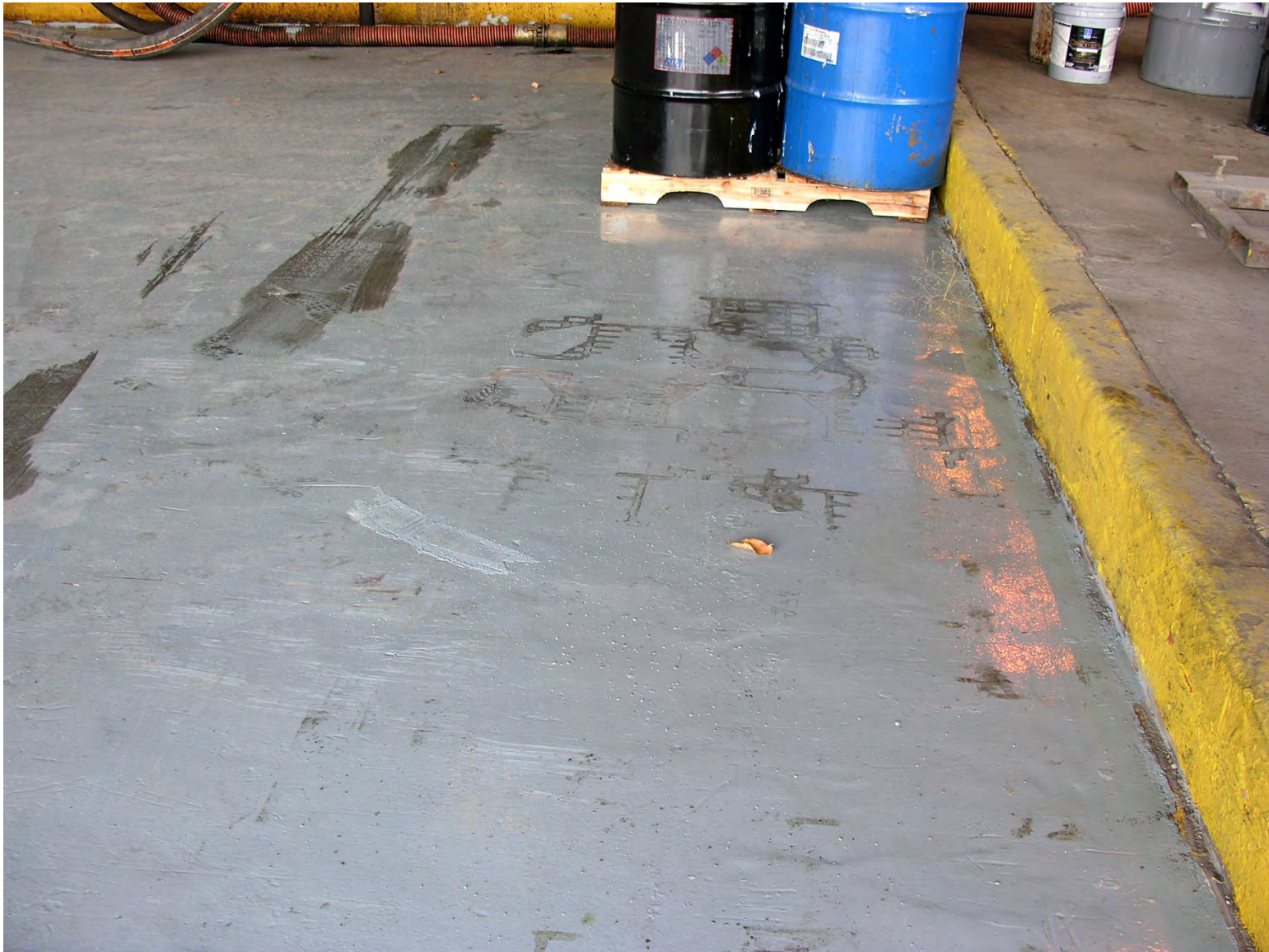
Closer View of Unloading Area #1 at Southeast Corner with Sump Trench in Background
