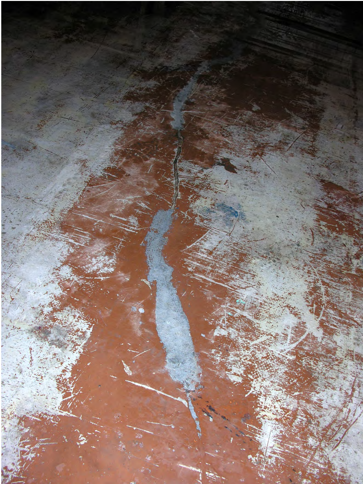
Aged Coating Repair of Slab Indicative of Acceptable Condition of Slab in General
