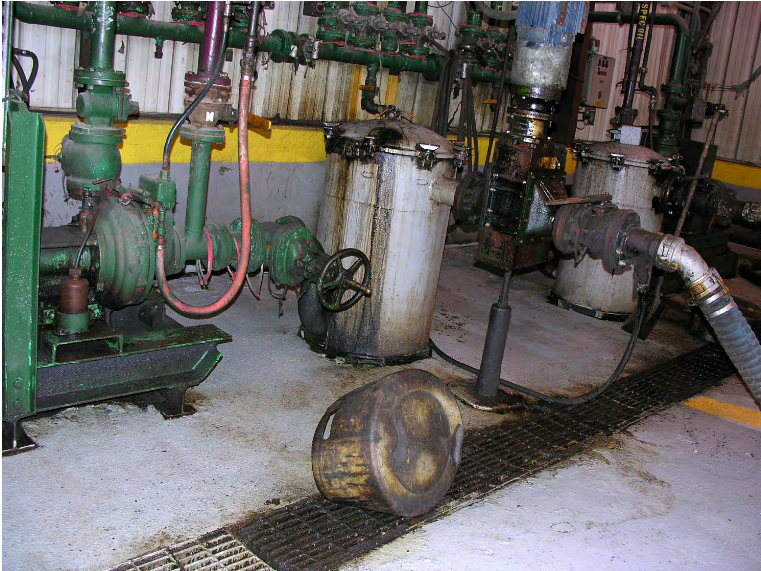
Pump Equipment at Unloading Area #2 Looking Southeast
