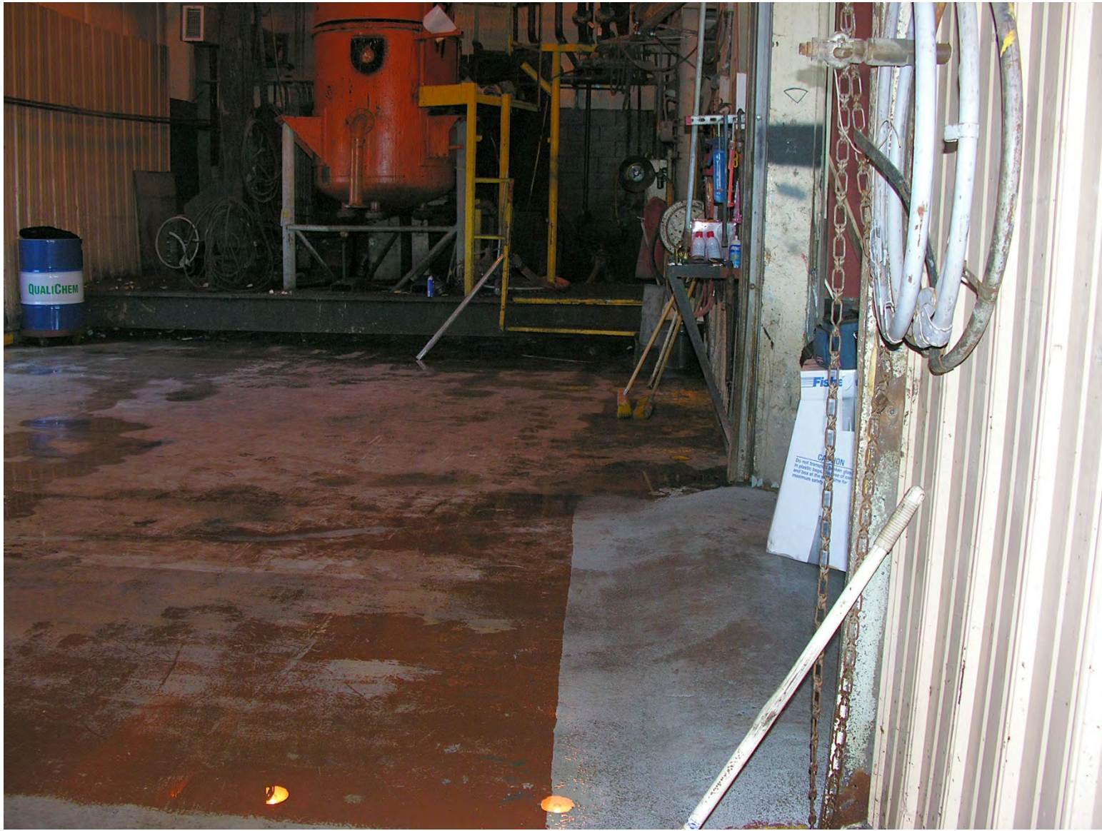
Earlier Photo at Speed Bump Entrance Curb Prior to Re-coating Showing Slab Coating In General in Well Maintained Condition
