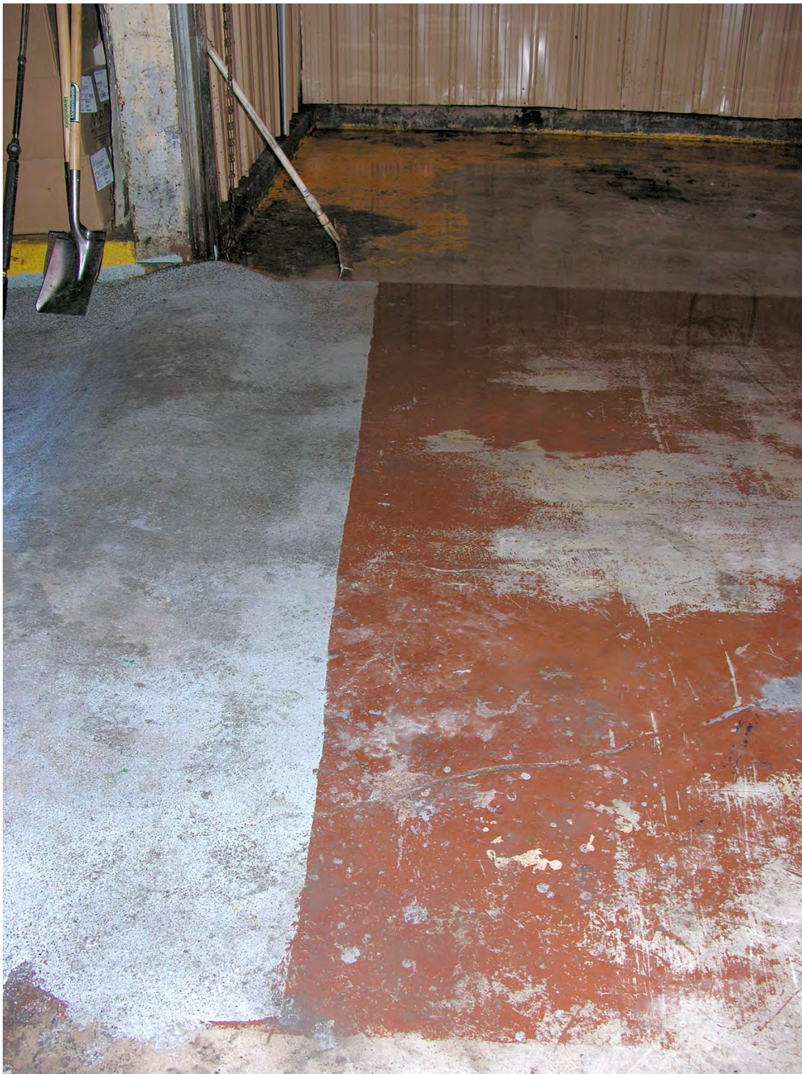
Alternate View of Speed Bump Entrance Curb and General Maintenance of Major Cracks to Acceptable Conditions
