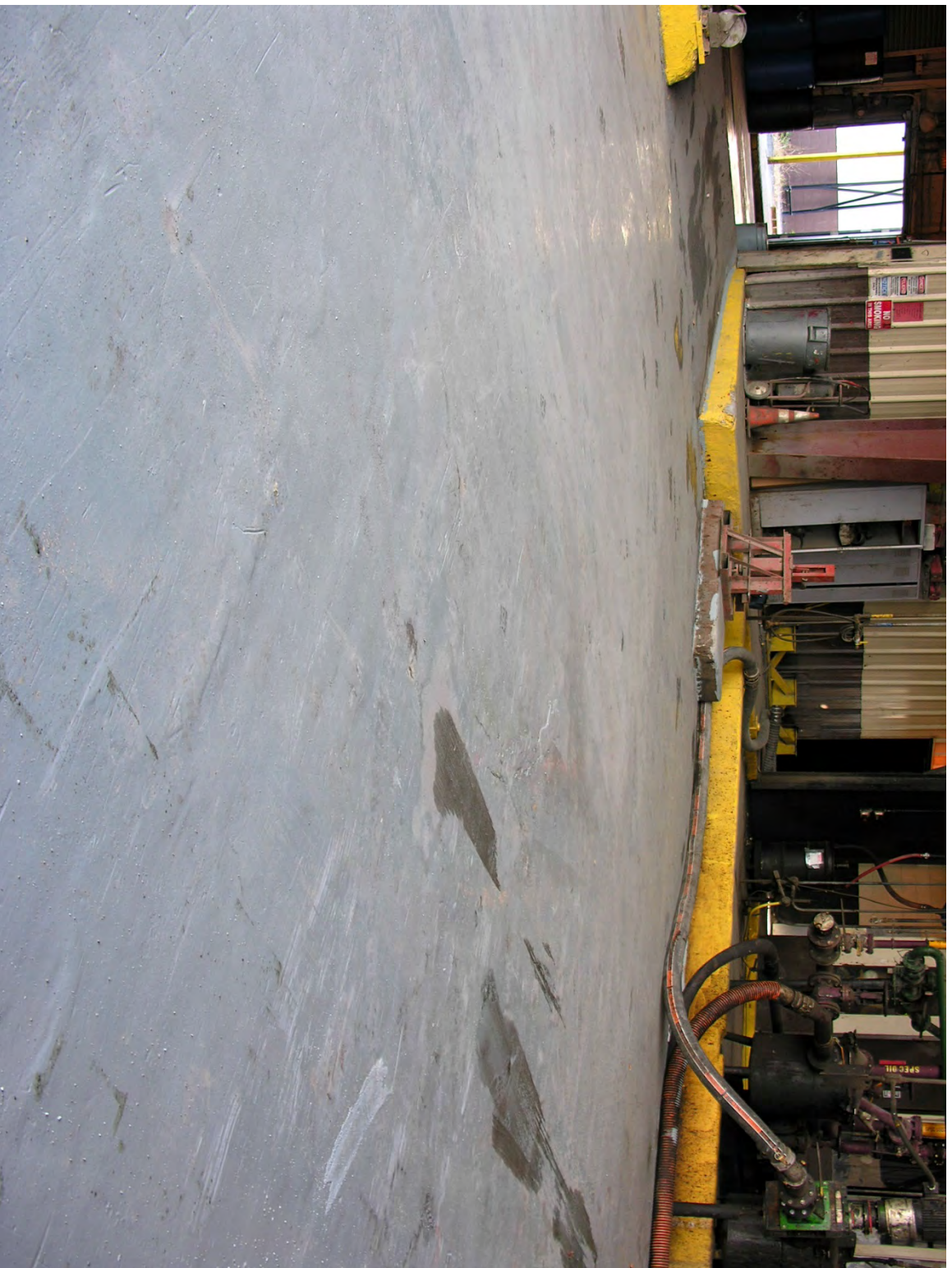
Closeup View of Unloading Area #1 Containment Showing Underlying Original Coating with Maintenance Re-coat
