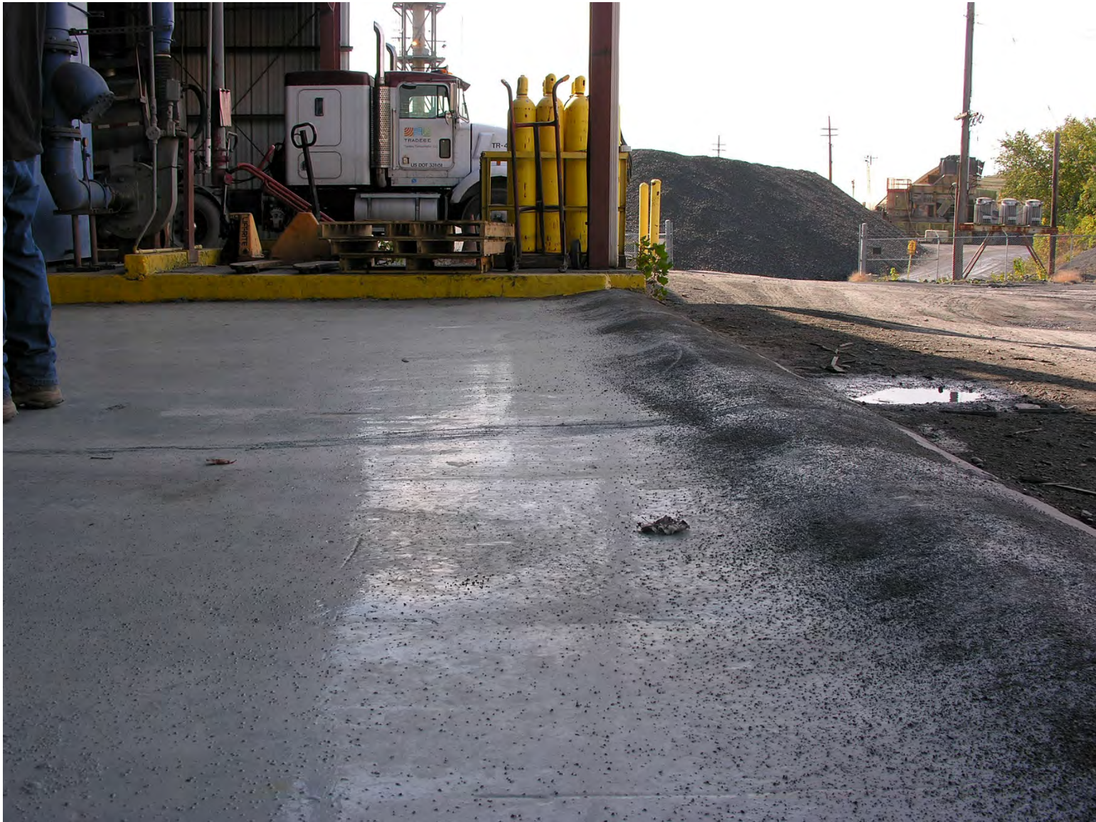
Unloading Area #1 at the Entry Berm Showing Maintenance Coat with Grit Broadcast for Traction
