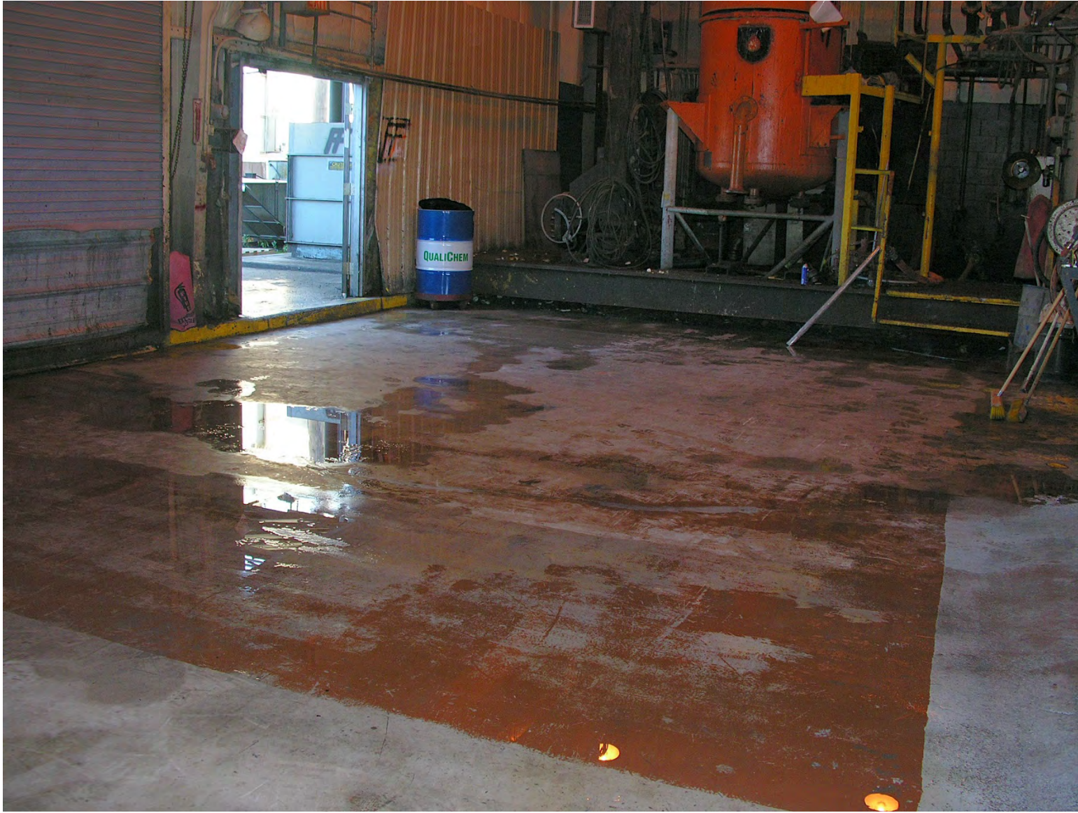
Earlier Photo Prior to Re-coating Shows Slab Coating In General in Well Maintained Condition
