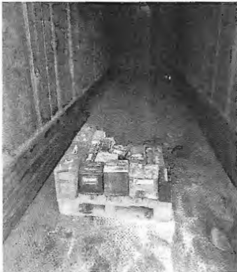
Photo 3: New Battery Storage Area
