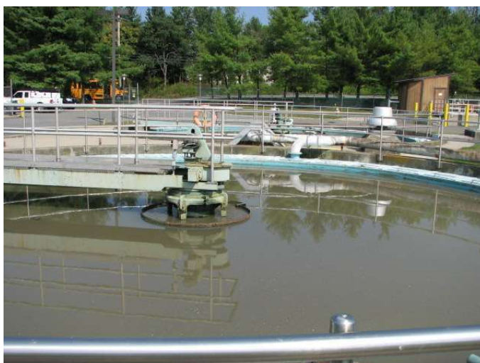
Figure 7: Secondary Treatment Clarifiers
