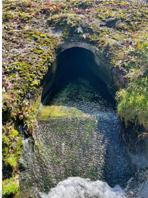
Outfall 001 (Source: Town of Cazenovia, NY-2A Application)
