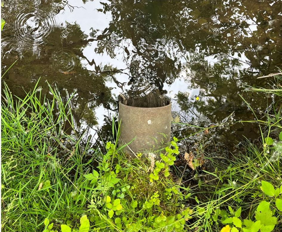
Image 1: Picture of the Outfall
